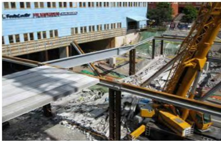
Figure 2.4: Same View as in Figure (2.3), After Collapse
