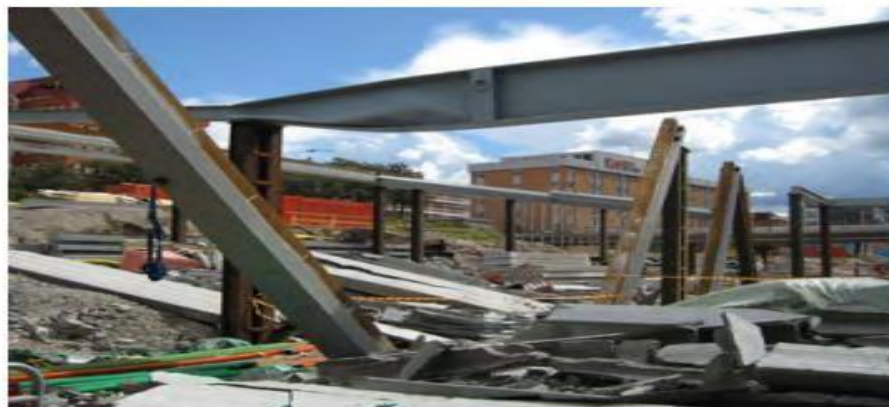
Figure 2.5: The Structural Collapse Was Caused by a Welded I-Girder That Was 1400 mm high.
